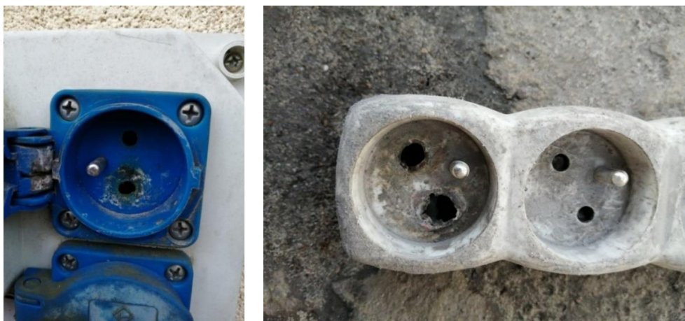
Fig. 5. Examples of the effect of improper use of electrical equipment
