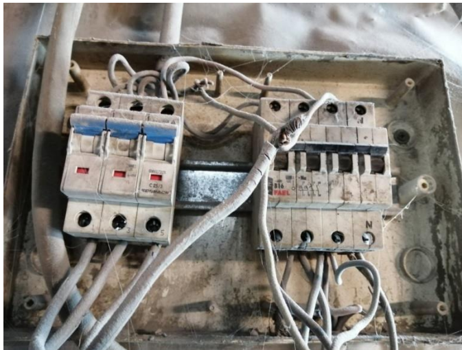
Fig.4. Improper installed current switchgear
